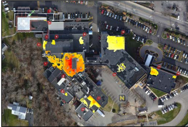
Colorized Moisture Hidden Inside Roof Insulation
